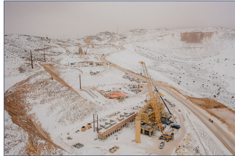
Pre-Screen & Tertiary Crusher
