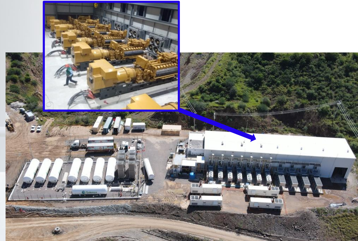
Santa Elena's 24MW LNG Power Plant
