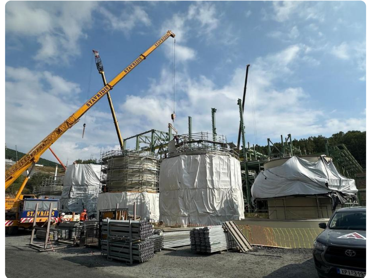
Tank farm at filtered tailings plant
