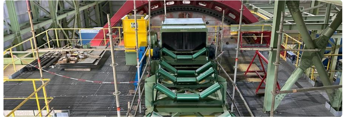
Process plant – sag mill feed conveyor
