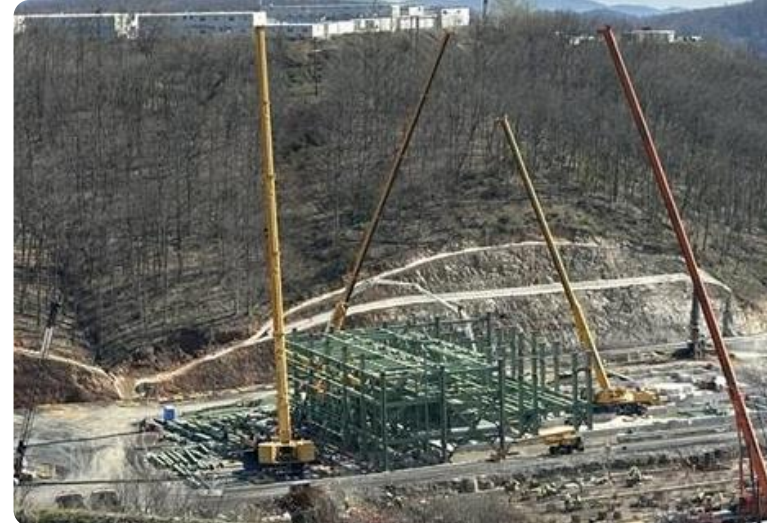
Filter plant facility overview
