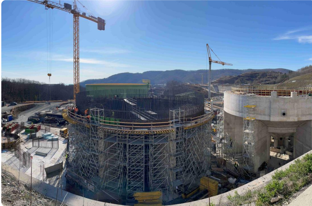
Thickeners – concrete works progressing on first two, and construction on third thickener has commenced.
